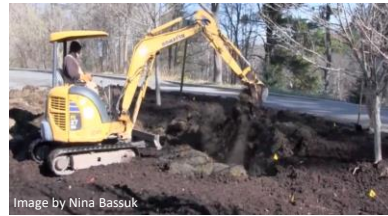
Yellow flags mark the root zone of an existing tree to be protected.
